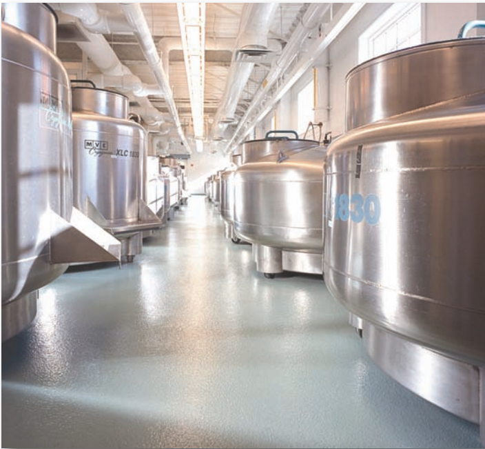
Stonhard floors protect areas around tanks in a cord blood storage area within Coriell Institute.
